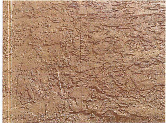
6.i Cracks in small areas
