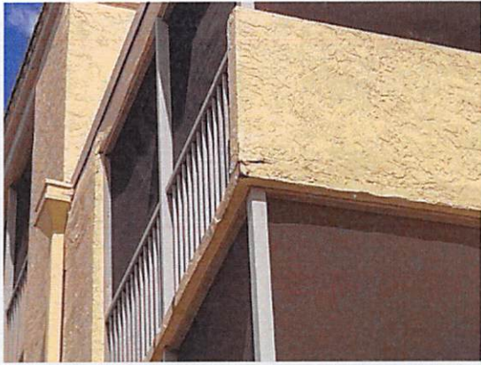
5.d Hairline cracks on walls
