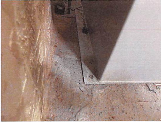
8.f Elevator machine rom
