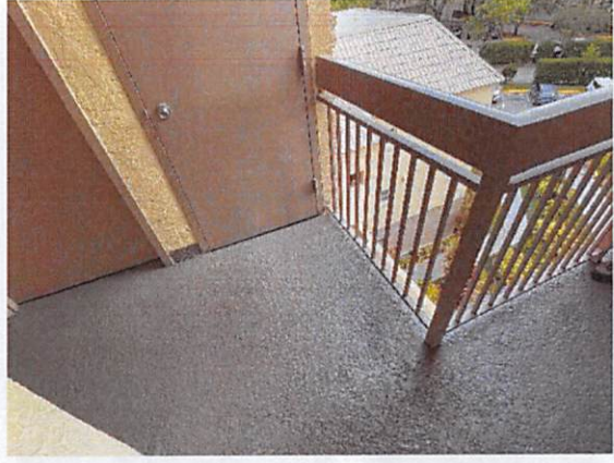
7.b.5 Guard rails in fair condition
