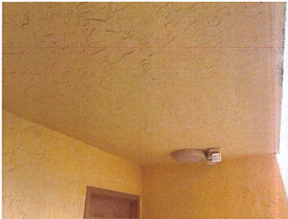
6.j Spalling in small areas.
