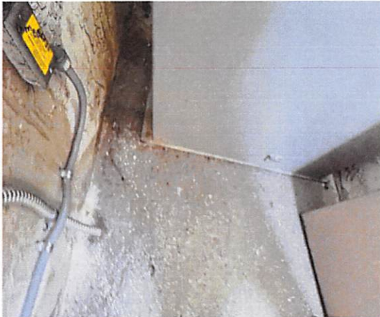
8.f Elevator machine rom
