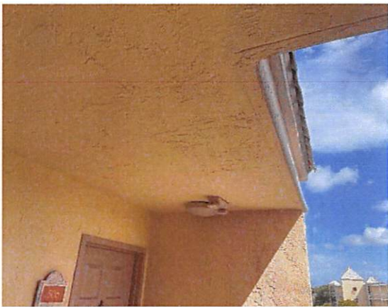
6.j Spalling in small areas.
