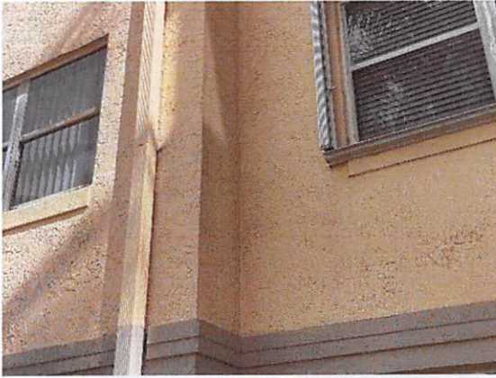
5.d Hairline cracks on walls
