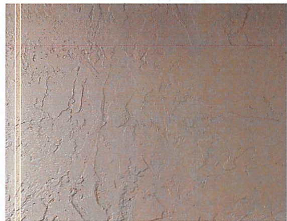
5.c Hairline cracks on stucco
