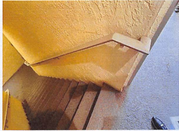
7.b.5 Guard rails in fair condition
