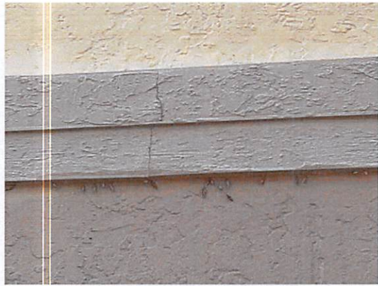
6.i Cracks in small areas
