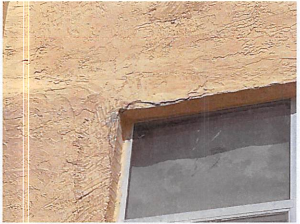
5.c Fine cracks on stucco
