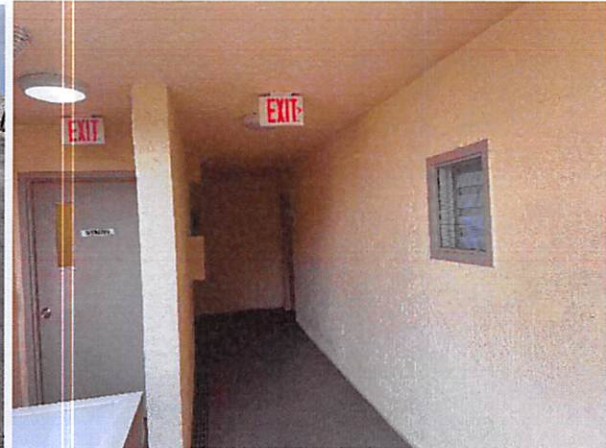
7.b.1 Floor system in fair condition
