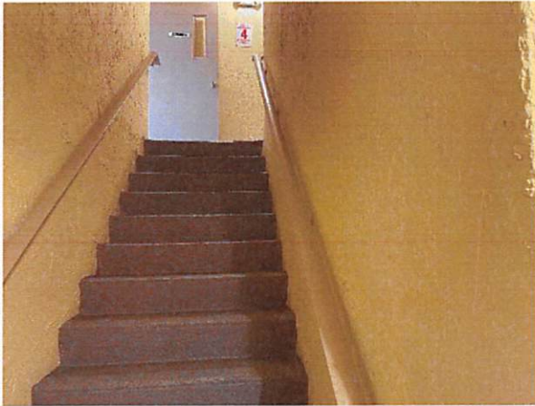
7.b.5 Guard rails in fair condition
