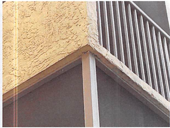
6.i Cracks in small areas
