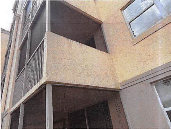
6.j Spalling in small areas.
