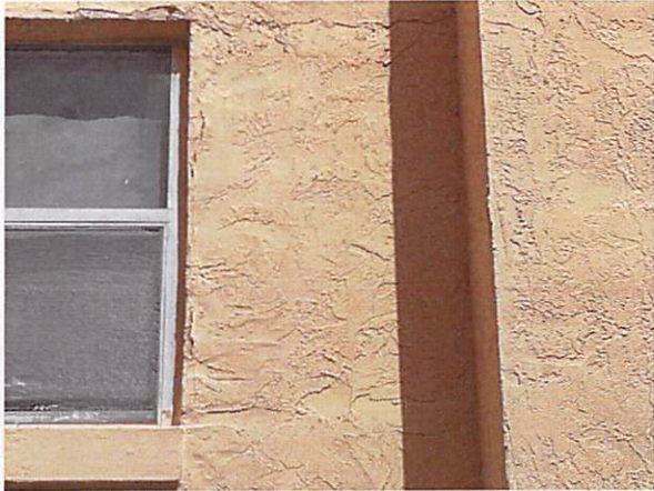
5.d Fine cracks on walls
