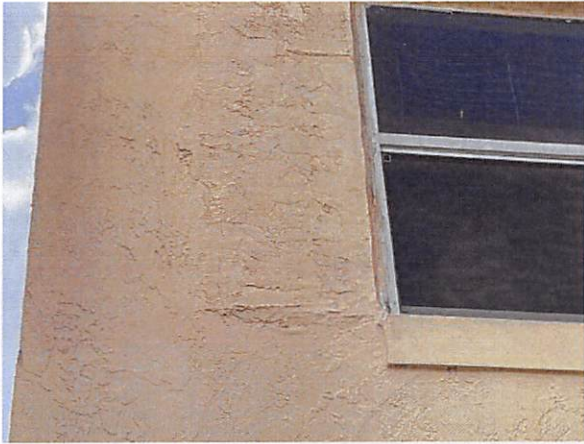
5.d Fine cracks on walls
