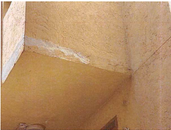
5.b Some areas present repaired cracks
