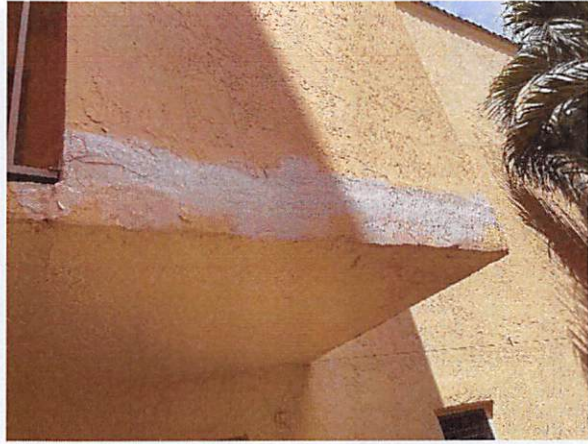
5.e Some areas present repaired cracks
