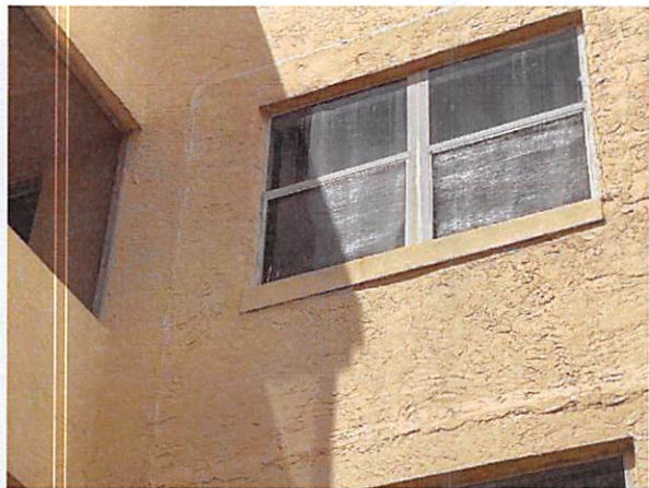
5.c Fine cracks on stucco
