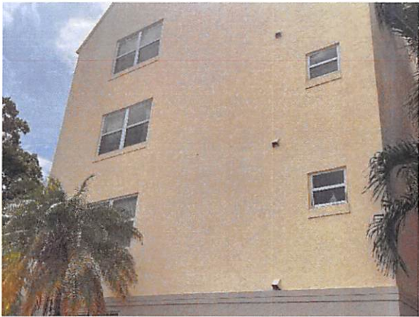
6.j Spalling in small areas.
