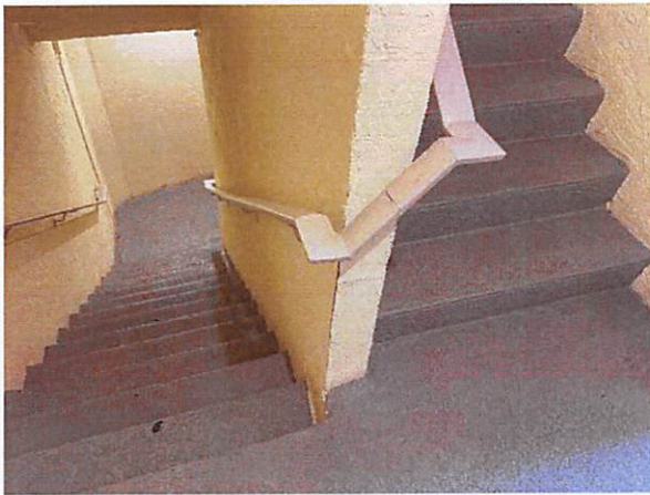
7.b.5 Guard rails in fair condition
