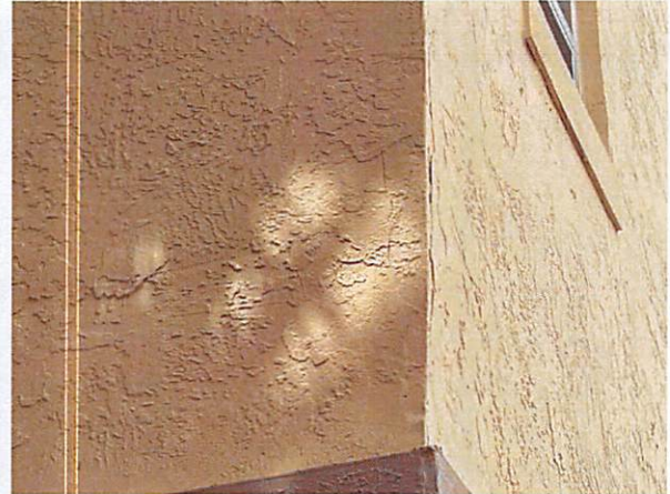
6.i Cracks in small areas
