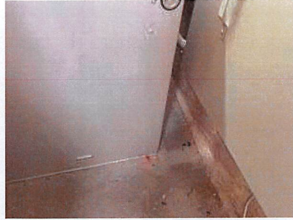
8.f Elevator machine rom
