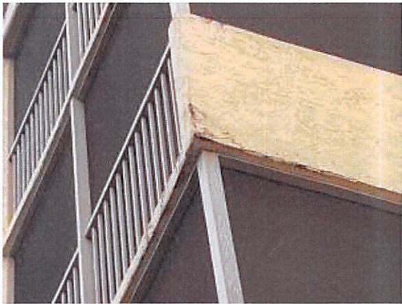
6.i Cracks in small areas
