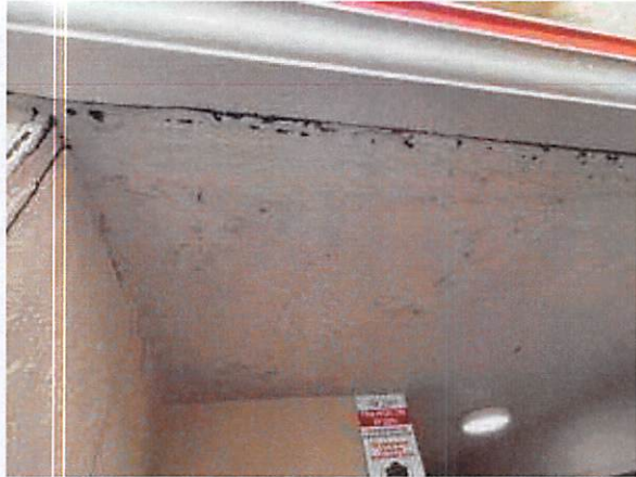
5.c Fine cracks on stucco
