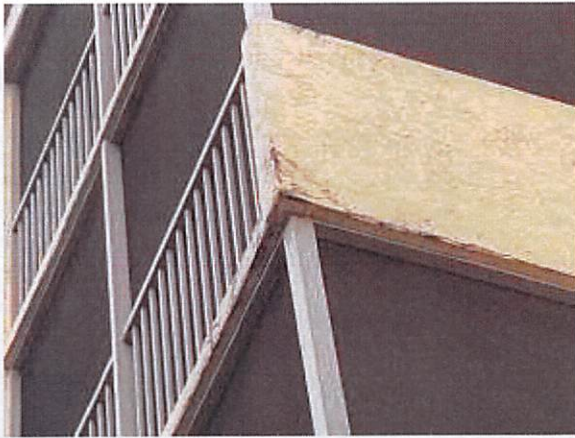
5.d Fine cracks on walls
